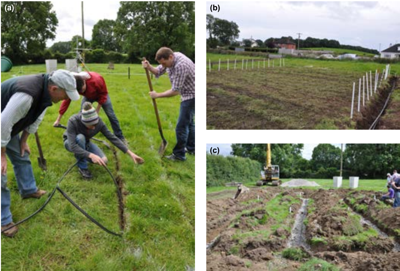
Figure 2.15. (a) Installation of DD tubing, (b) final DD installation at Site B and (c) installation of LPP at Site A.
