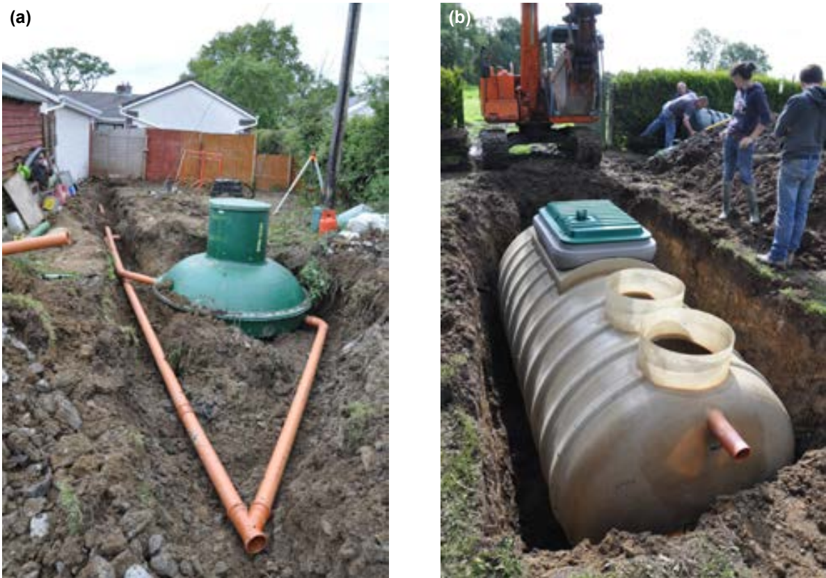
Figure 2.16. Packaged treatment plants: (a) extended aeration process at Site A and (b) media filter at Site B.
