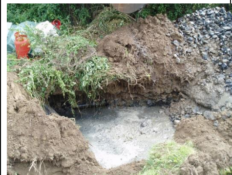
Old septic tank percolation area was flooded
