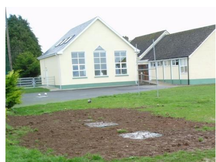
Secondary treatment replaced the septic tank for school extension
