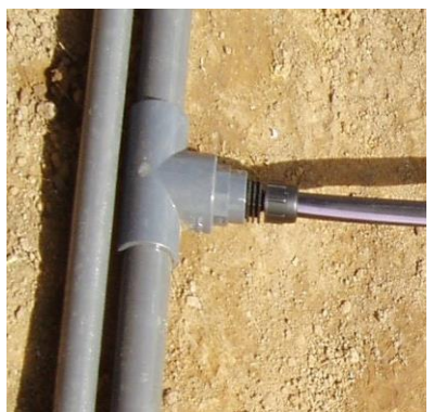
Dripline connection to PVC manifold in a network arrangement
