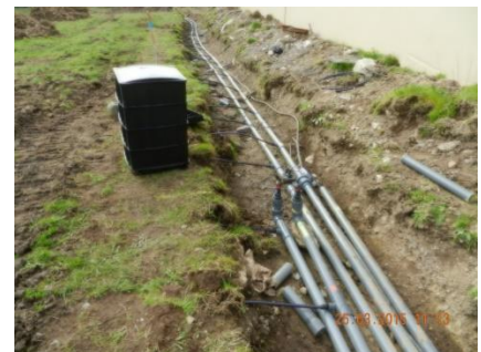
PVC manifolds to multiple cells with solenoid valve controlling sequential 6 zone dosing.
