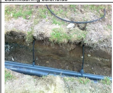
Connections to PVC manifold by Ashtecs
