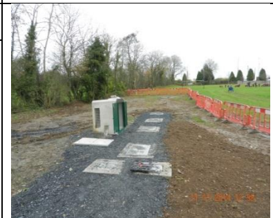
secondary treatment system
