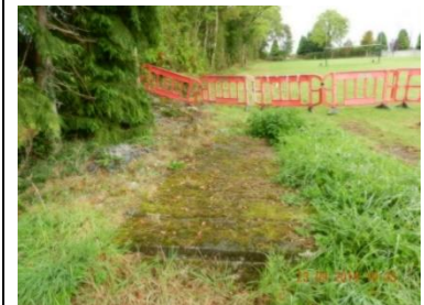
Existing septic tank was polluting the adjoining stream.
