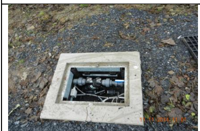
Drip headworks with 130 µ filter and backwashing solenoids
